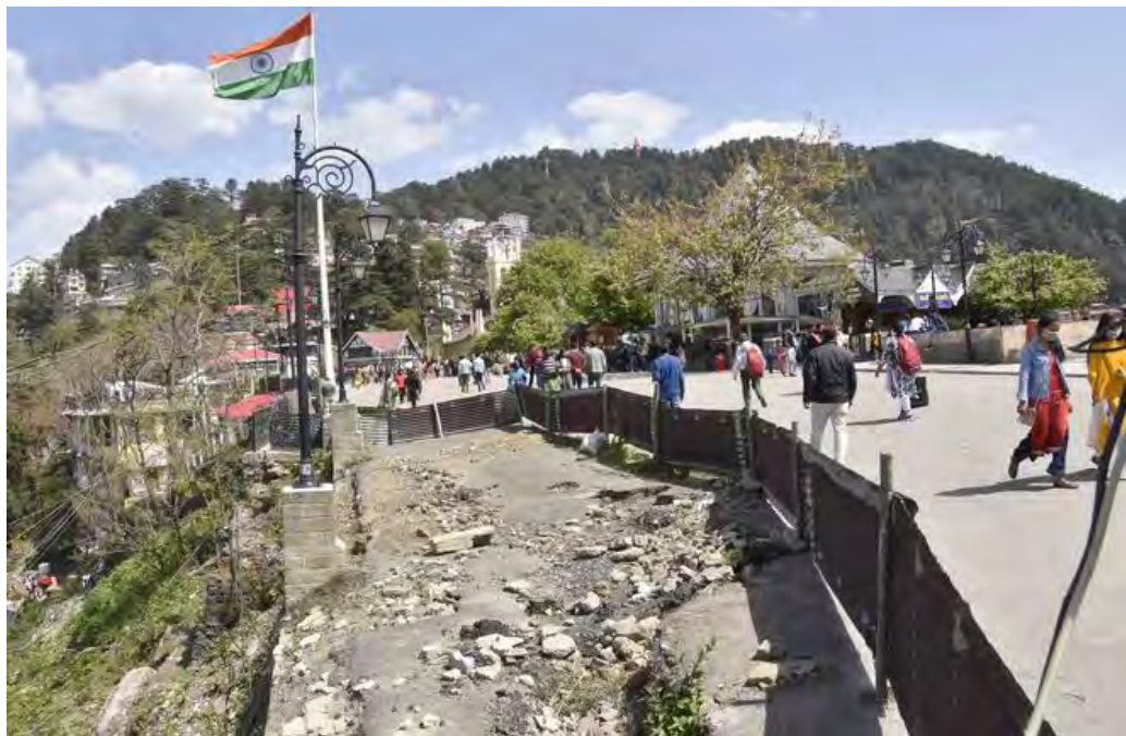
Sinking Area near the Ridge, Shimla
